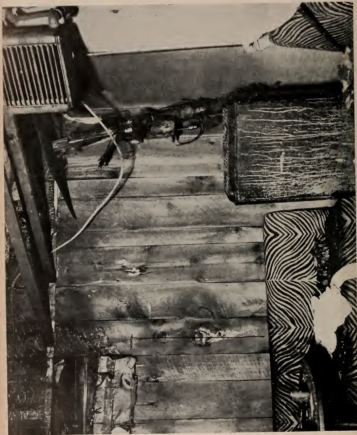
Northwest Corner of Melody Lounge, Where Fire Started.
